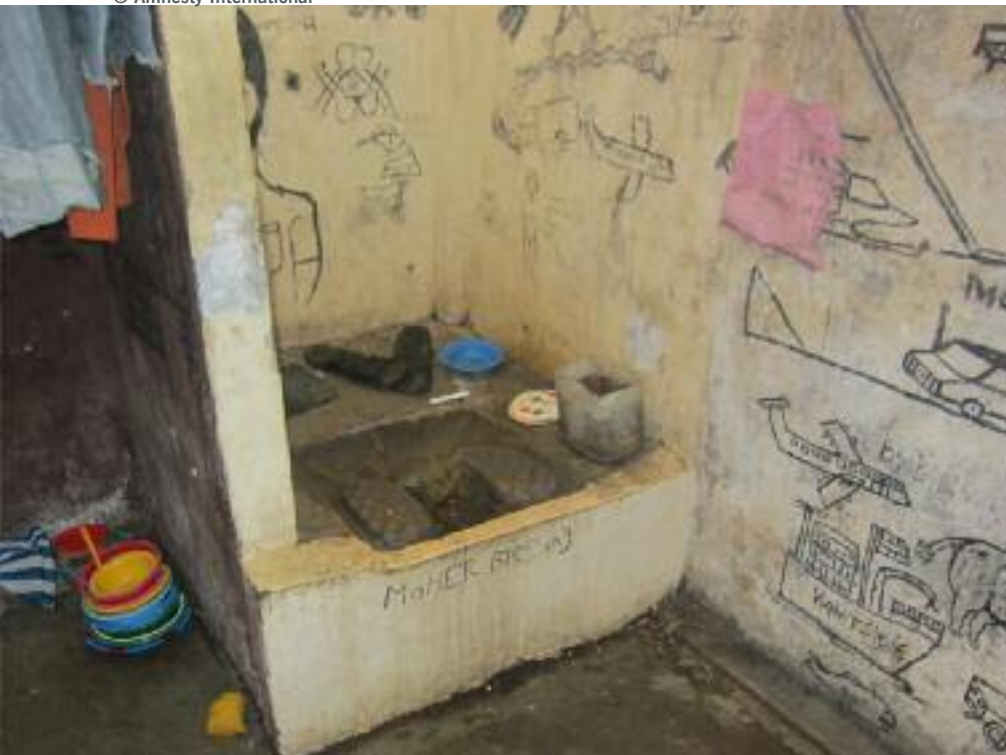
Top: The communal bathrooms at Monrovia Central Prison are dark, wet and dirty. There isn't enough water for the inmates to bathe with any regularity, and there is no plumbing.
